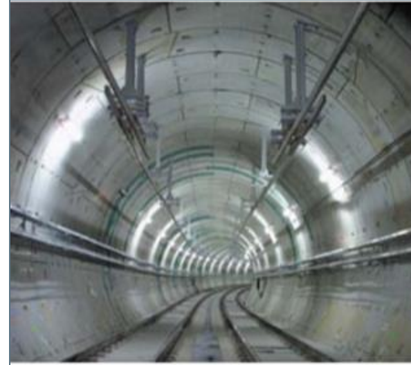
Rigid tunnel catenary
